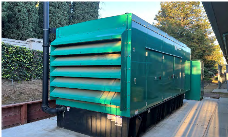
D. Civic Center Emergency Generator Project
