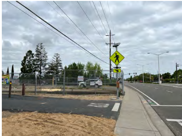
J. Pedestrian Crossing Lighting System Installation on O'Hara Avenue at Trail Crossing Project
