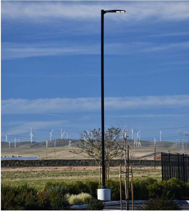
Typical Single-Head Parking Lot Lighting
