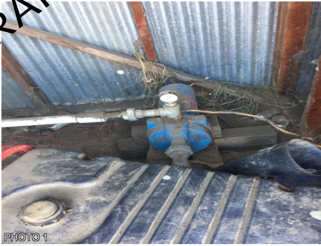
PHOTO 1 VIEW OF WELL PUMP LOCATED IN SHED.
