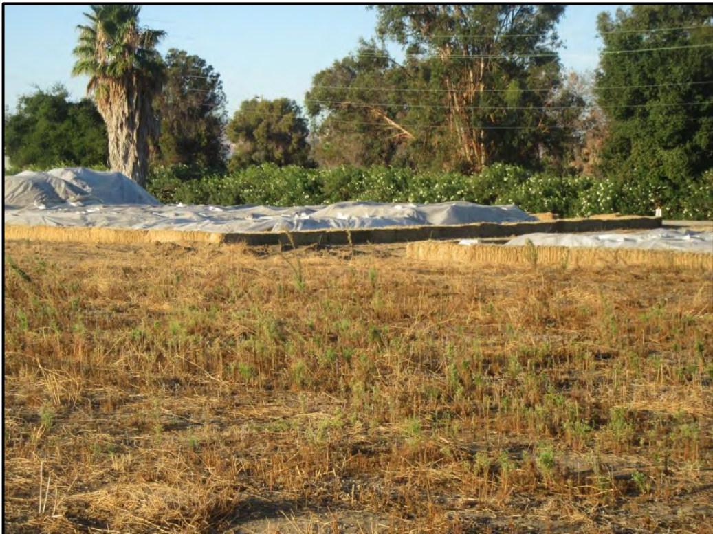
Location of ongoing soil remediation in the north part of the site, looking southwest; 11/02/18.
