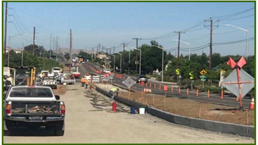
Laurel Road west of Rose Avenue is pictured above and Laurel east of Rose is pictured below as construction continues on pace to finish by the end of this summer.
