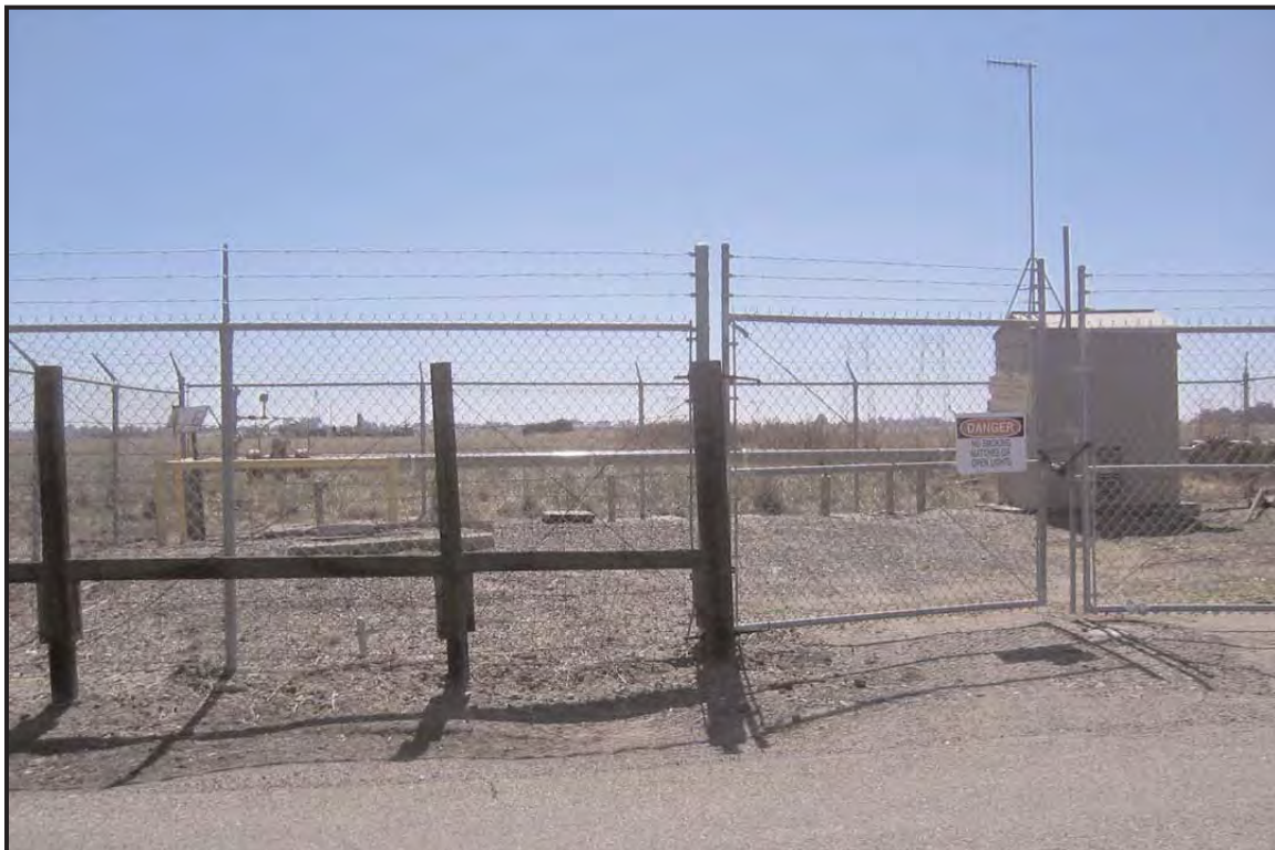
Photograph 6. An existing natural gas pump station along the east side of Jersey Island Road.
