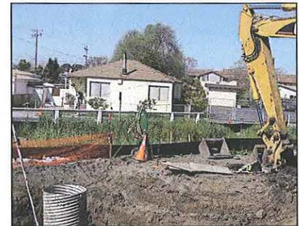
CME WILL WORK WITH THE CONTRACTOR TO MINIMIZE IMPACTS TO RESIDENTS DURING CONSTRUCTION
