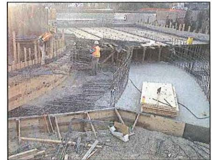
MANY UTILITIES WERE RELOCATED DURING THE BART EXTENSION TO SFO IN SAN BRUNO
